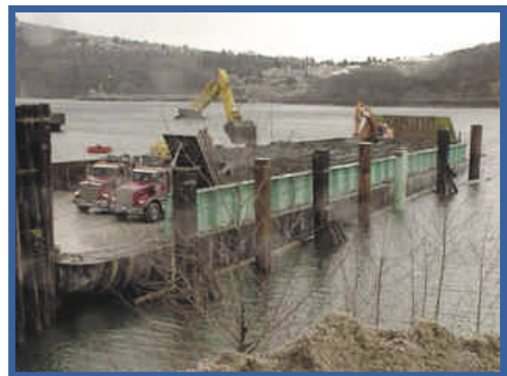
Dredgeates and excavated soils from construction form the bulk of materials disposed at sea.
