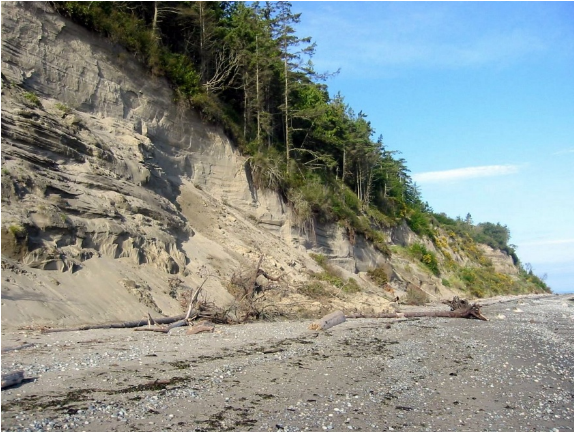
Figure 4. Eroding bluffs at Fort Worden in Port Townsend.
