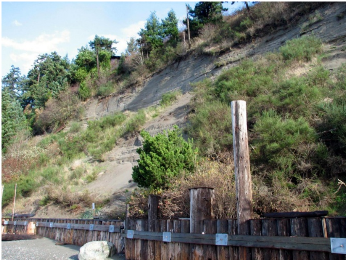
Figure 17. A timber pile bulkhead at the base of an eroding bluff in Snohomish County.
