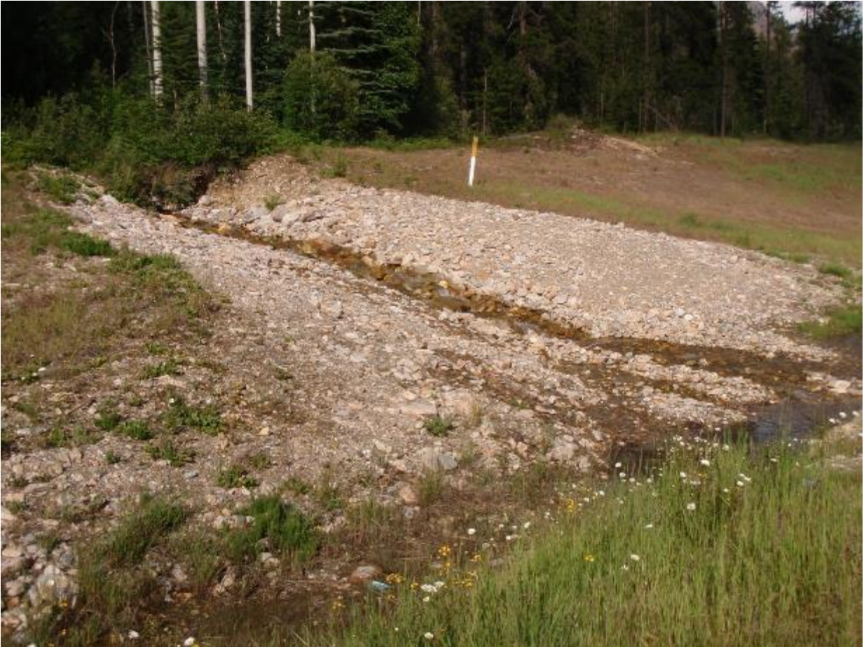
Figure 23 Extreme damage to a stream crossing the TMP ROW. Virtually all habitat capacity has been destroyed in this small stream located west of the Alberta-British Columbia border adjacent to the highway and crossing the TMP ROW. Under any-other circumstances it is incomprehensible that such destruction would be allowed to take place in a CRA-fisheries stream, or a stream that flows into CRA-fisheries waters.
