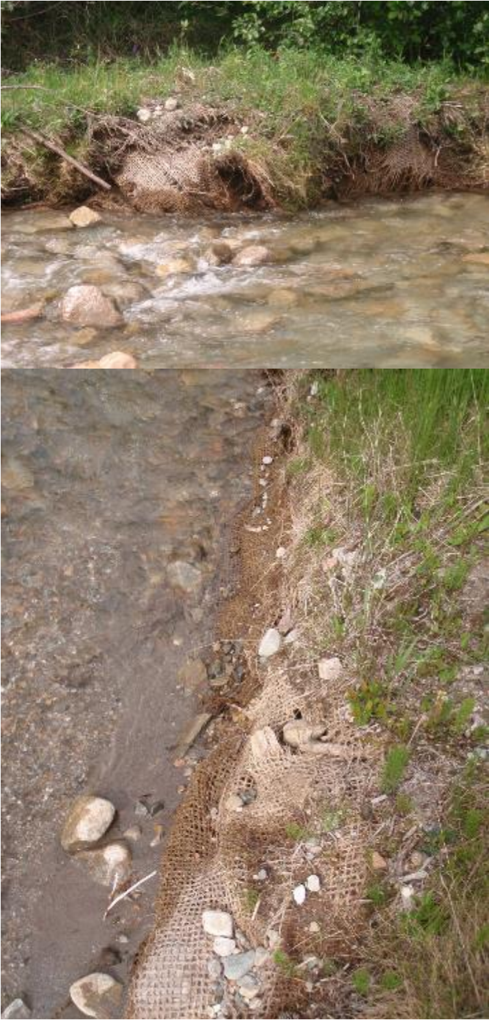
Figure 21 Coco-mat debris remaining at Clairvaux Creek from the TMP Anchor Loop construction.
